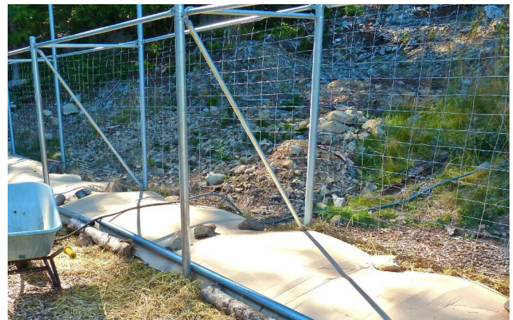
The poles in this area would not go deep enough as it was too rocky so Phil engineered triangular cross bars to stabilize them.
