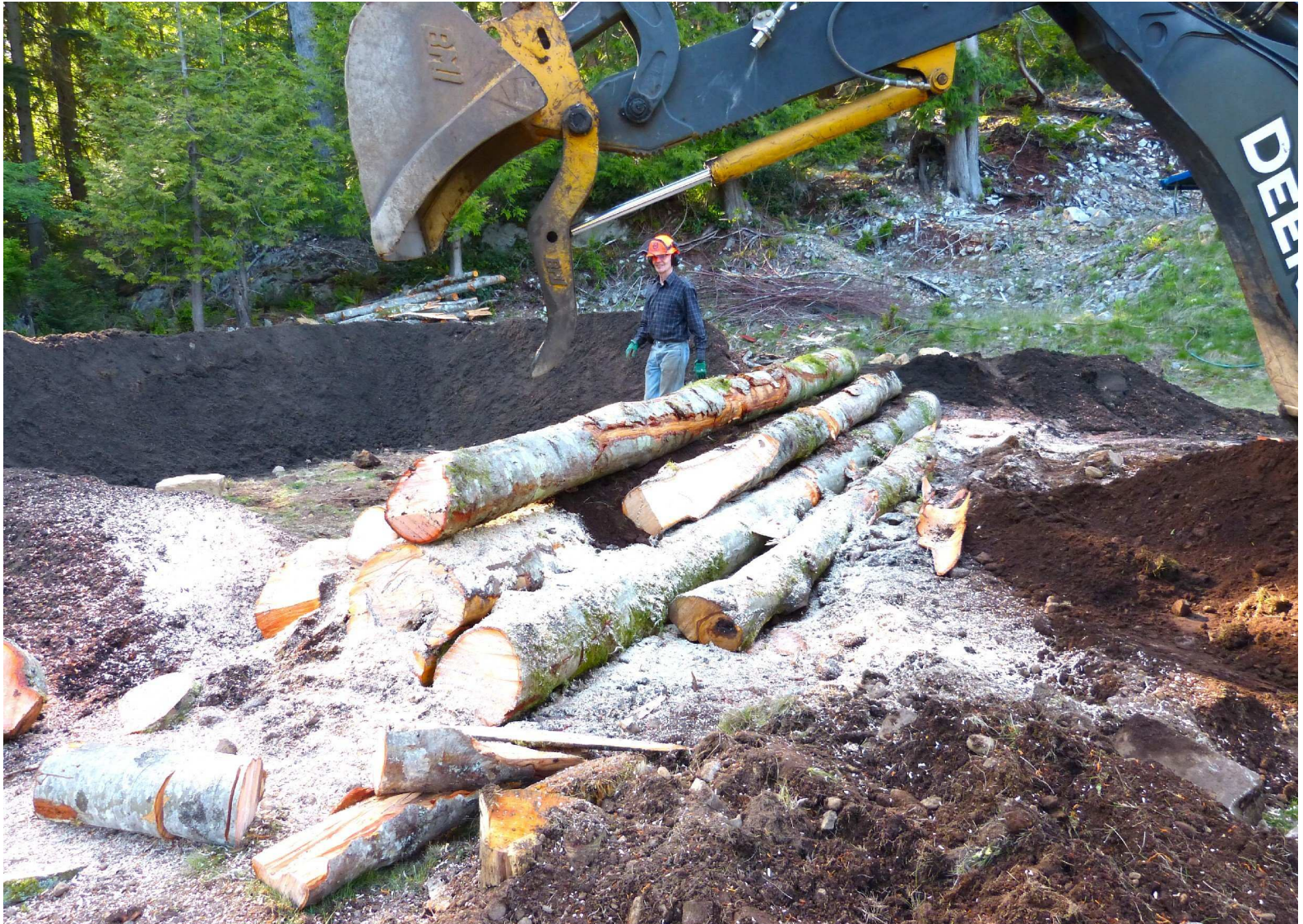
A shallower slope There are still quite a few more logs to add here, but it doesn't get any higher.
