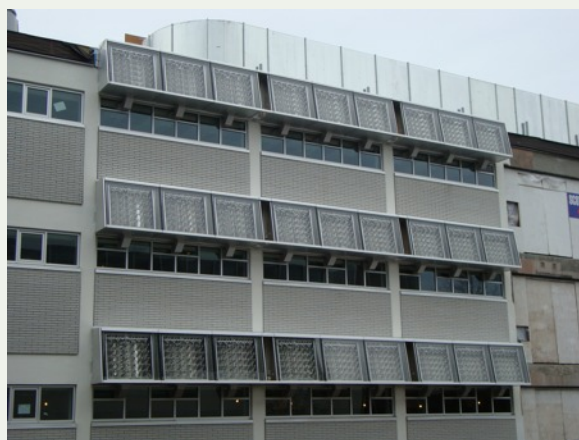
The second installation is underway at the newly-renovated UBC Biological Sciences Complex.
