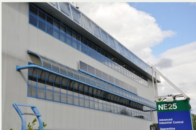
The Core Sunlighting system installation (completed) on BCIT campus in Burnaby.
